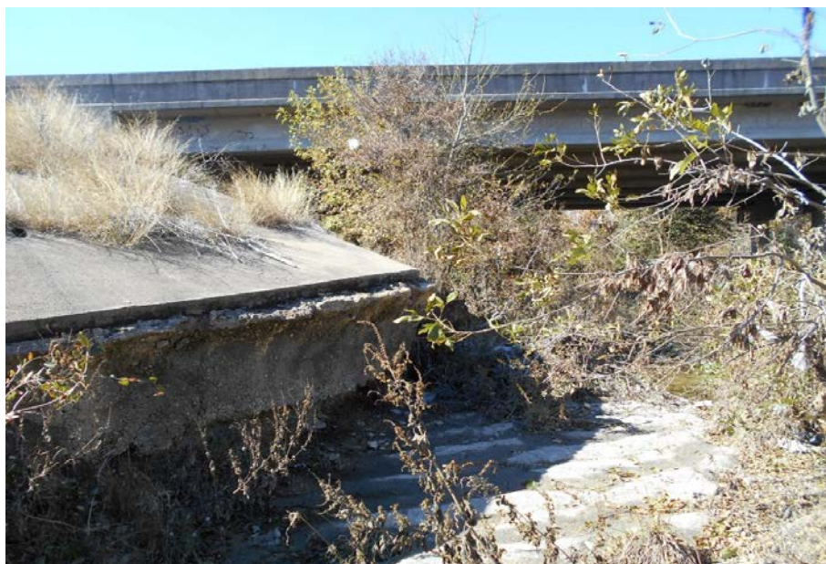
The downstream bridge abutment for the Roy Reynolds Bridge. Nolan Creek is eroding/undermining the concrete abutment.
